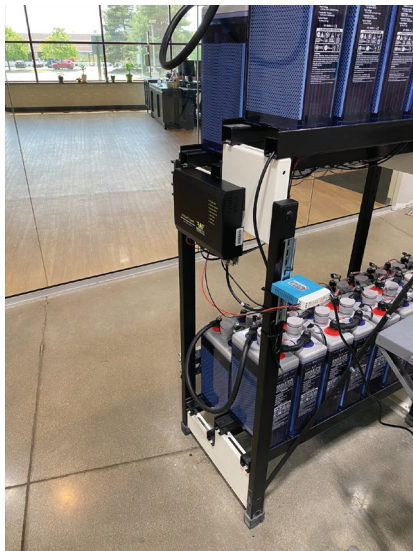
X Bad angle, not showing enough of the batteries
