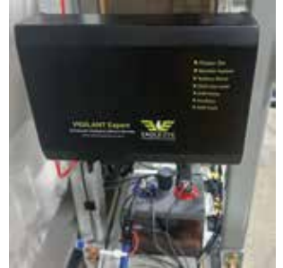
Battery Monitoring Systems
