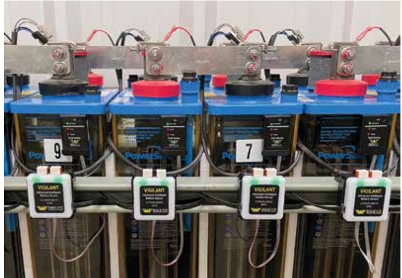
VIGILANT® Components Installed
