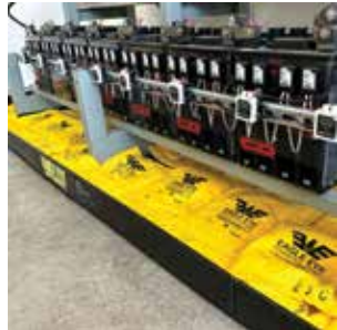
Battery Spill Containment
