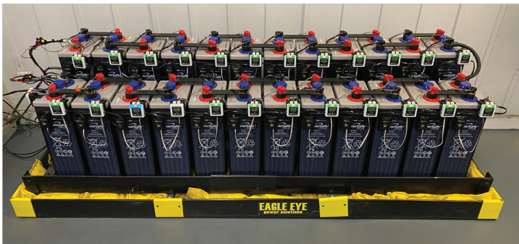
Vigilant Installation to Flooded (VLA) Cells
