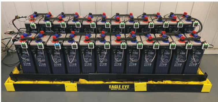
Vigilant Installation to Flooded (VLA) Cells
