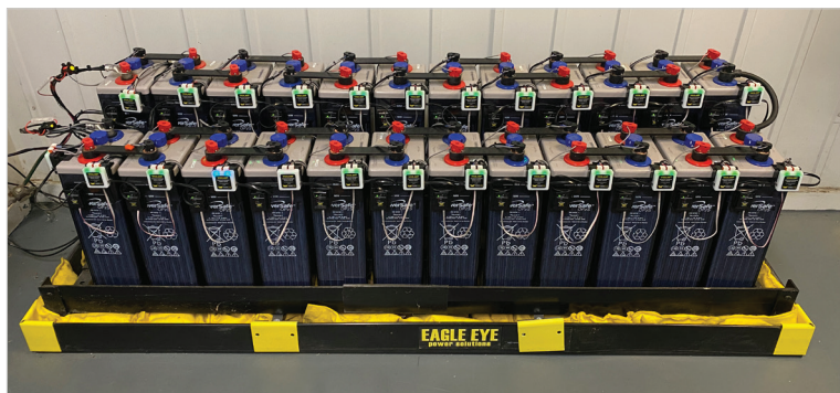
VIGILANT Installation to Flooded (VLA) Cells
