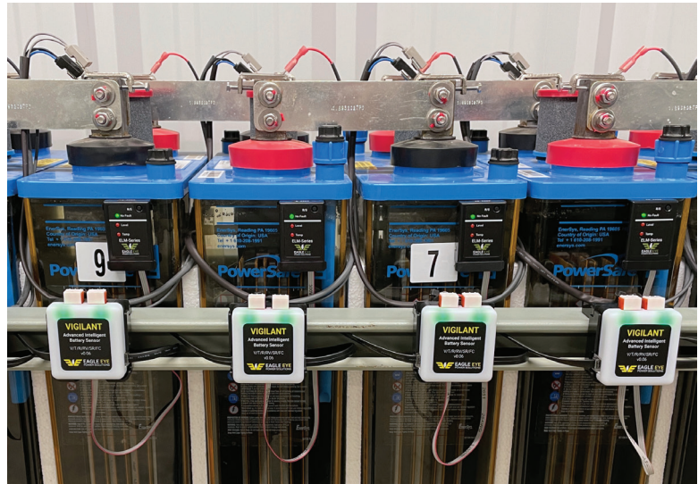
Vigilant Components Installed
